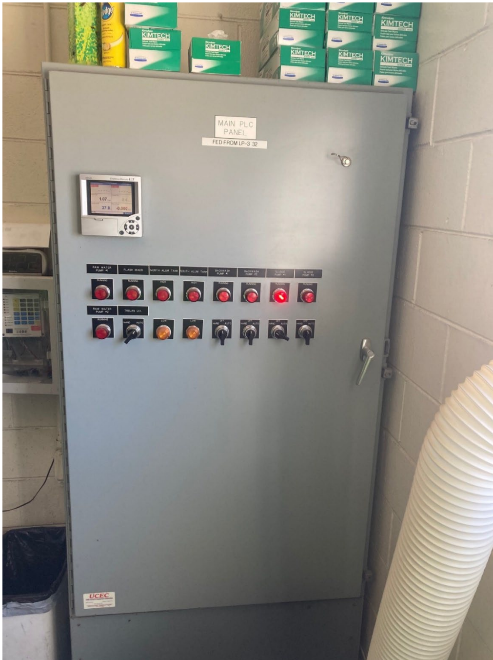
Figure 2. Programmable Logic Controller - Main Plant Facility
