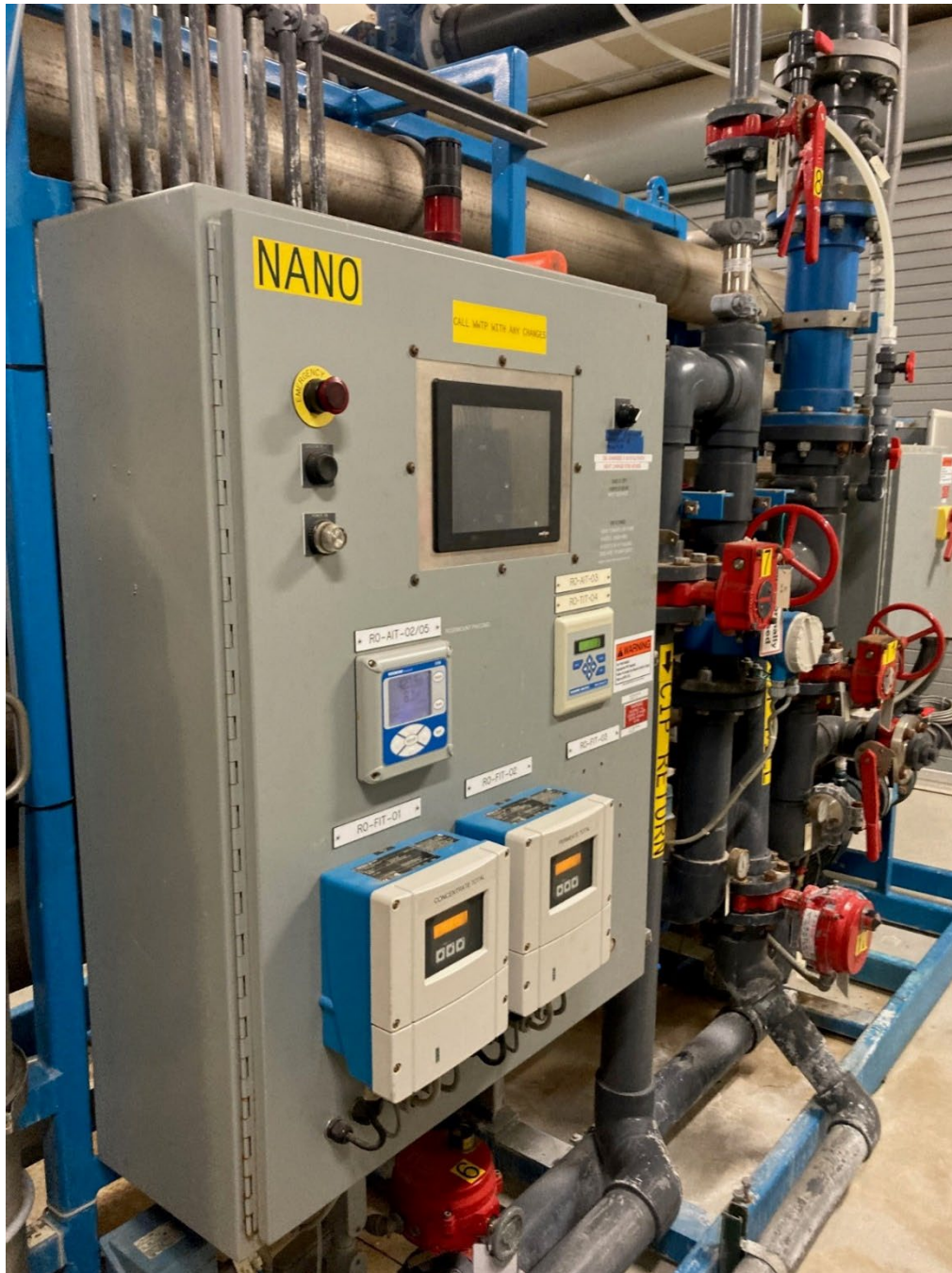
Figure 1. Programmable Logic Controller – Nanofiltration Facility
