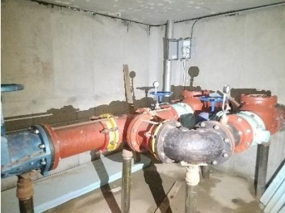
Image 2: Lift Station Valve Vault
